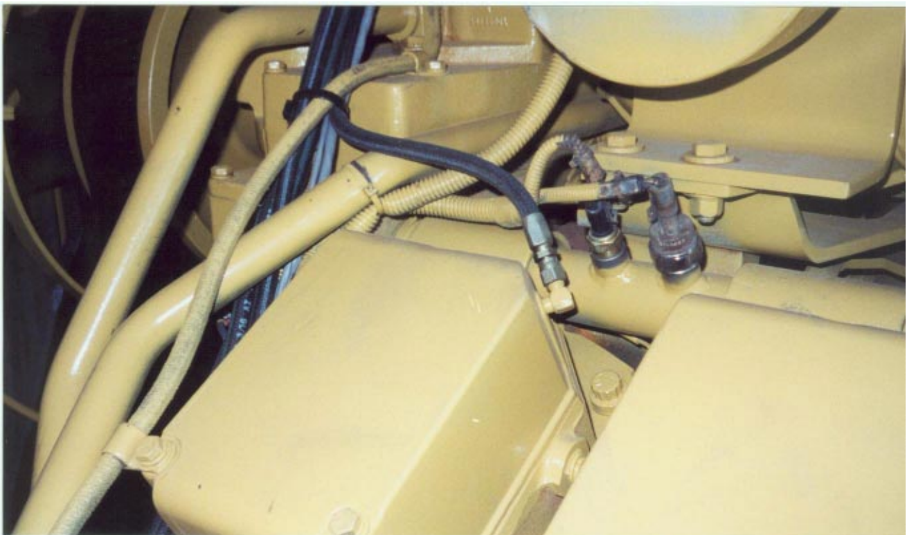
(Bottom) This is the Crankcase Pressure pick off point on the valve cover of a KTTA 50 Cummins Diesel. The pressure line runs from the Engine Saver® to the valve cover.
